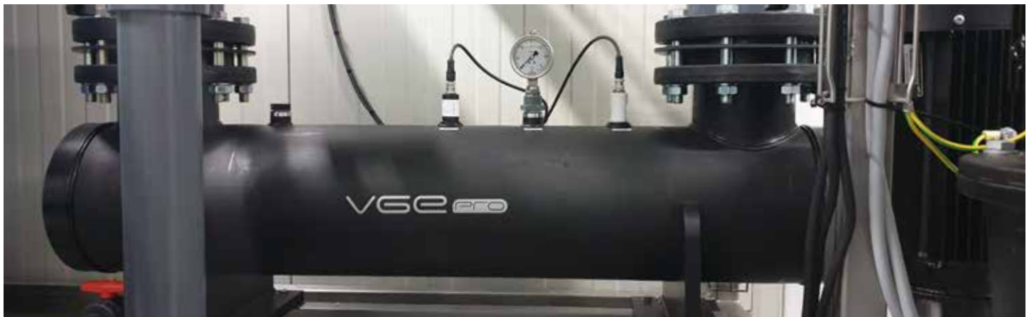
Drinking water - Libya - HDPE 600-225
