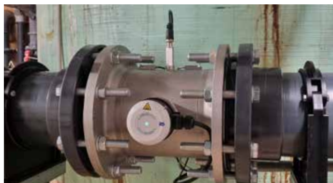
The Netherlands – Swimming pool and Spa - INOX MP 2000-219
